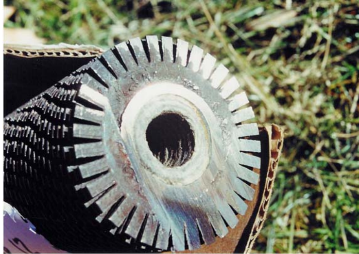
Figure 1 Heavy Deposit in HP Superheater Tube after Cycle Contamination with Brackish Water
